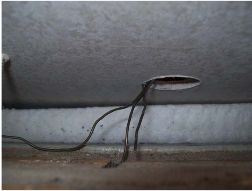
Figure 6: Thermocouples in weephole cavity and in cavity between cement sheet and brick wall.
