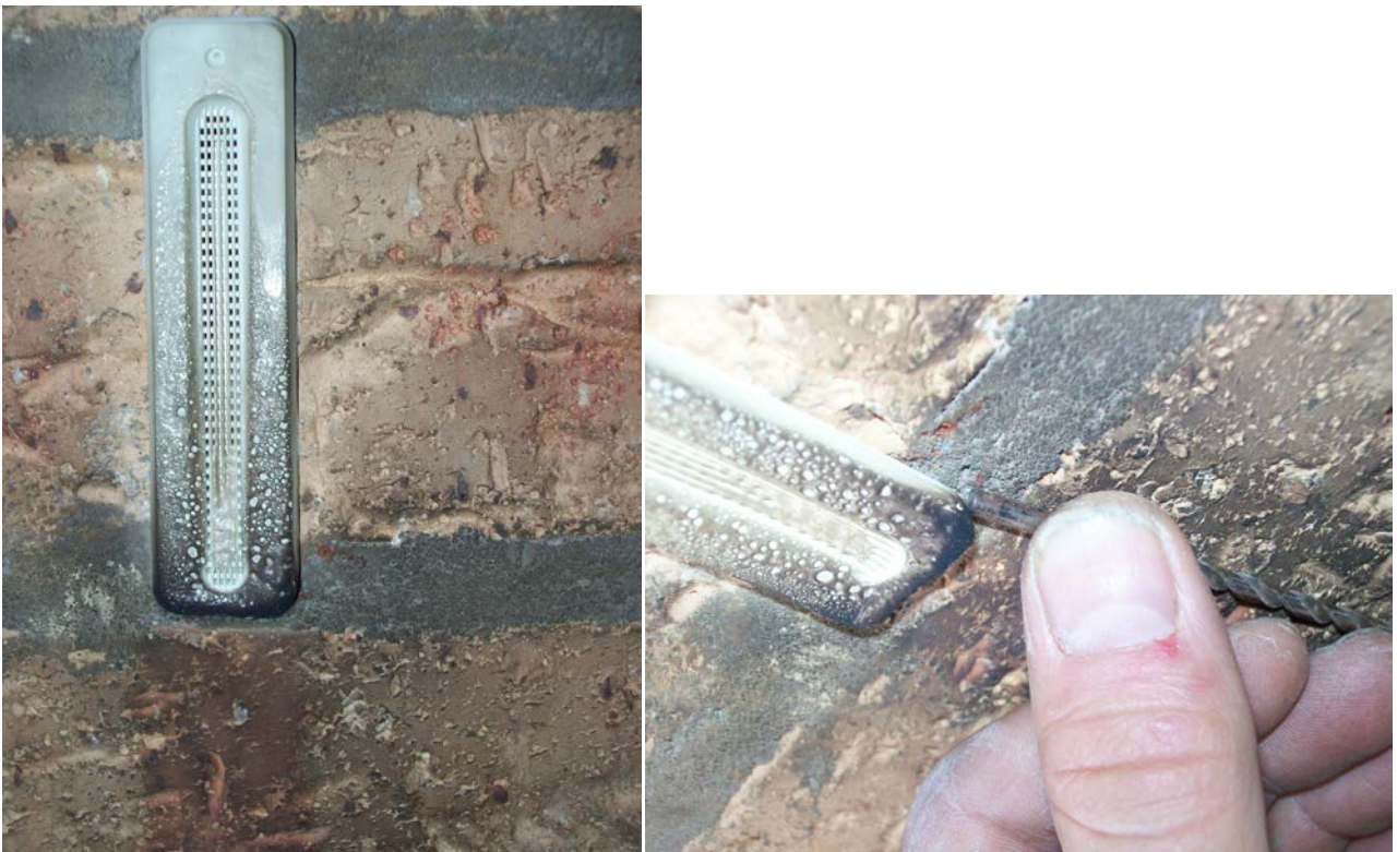
Figure 13: Post test Weepguard inspection.
